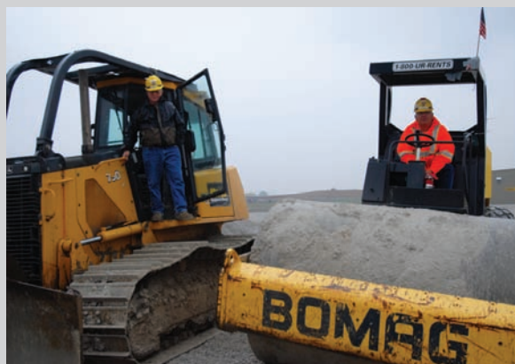
Dozer and roller operators Mike Dietz, left, and Don Rakers are part of the team of 165 operators building the new power plant.
