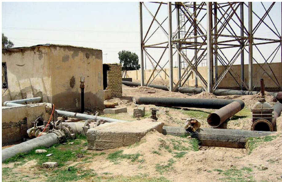
Ruins of the Safwan water plant, since restored by Bechtel
