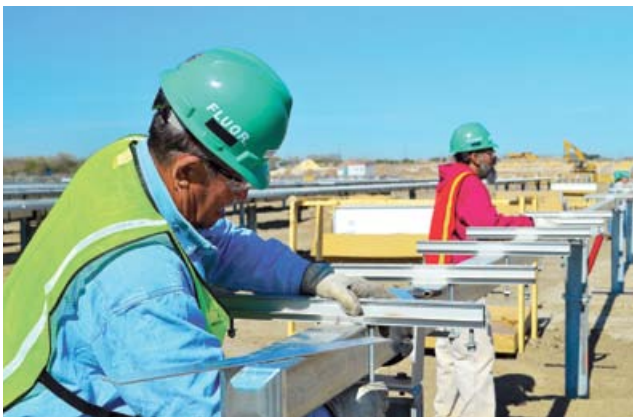
Fluor built a 30-MW PV project for SunEdison at a San Antonio Water System water treatment site.
