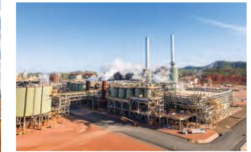
Yarwun 2 Alumina Refinery, Australia
