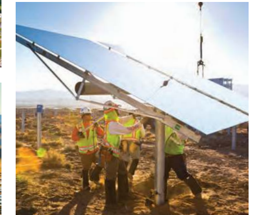
Ivanpah Solar Electric Generating System, United States
