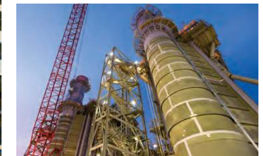
Russell City Energy Center Power Plant, United States
