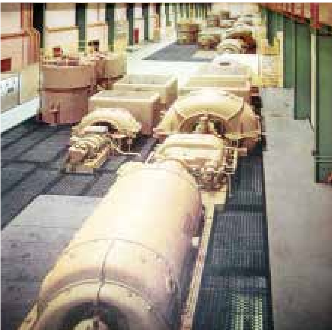
Reheat gas turbine hall. Brown Boveri’s two-shaft inter-cooled, reheat gas turbine power plant in Port Mann, Vancouver, BC, Canada. Note the four 25MW units lined up in a row along the turbine hall. The first unit is shown in the foreground with the generator connected to the low pressure train on the right and high pressure train on the left. The two vertical cylinders on the left are the LP and HP combustors.
