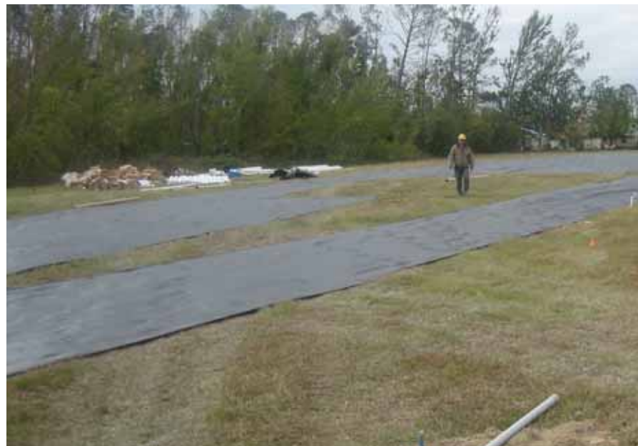
Photos 4 & 5 | Part of the solution was an application of up to 4 layers of geotextiles and aggregate, with just one layer applied to the stronger sites and perhaps all 4 layers needed for the softer sites.
